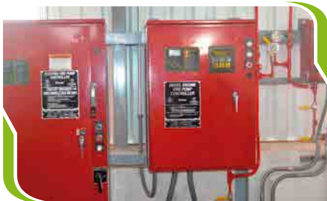
Paneles arranque bombas
